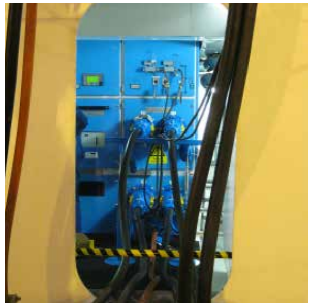
Picture 2: Example 11kV plugs for cruise vessels, (the same type can be used for 6.6kV cruise vessels), up to 20MVA power demand
