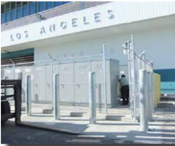
Picture 6: SSE substation at the Port of Los Angeles
